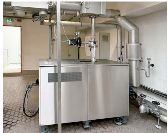
Depending on the running time, this system generates up to 175 MWh per year in a very small space. The amortisation time of the installation is then less than three years. Including all maintenance costs, over 270,000 Euros could be saved in 10 years.
