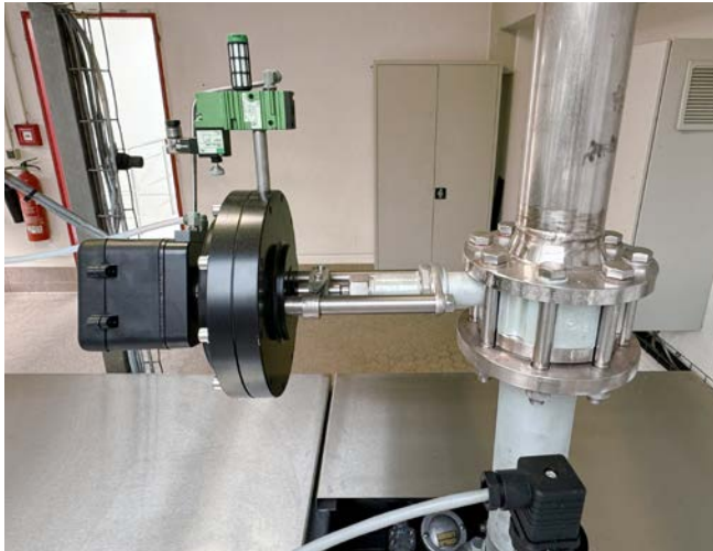
The DN80 sliding gate valve (15 kg) is more compact and lighter than each of the two previously installed globe valves (together approx. 170 kg).
