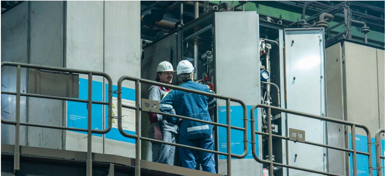
The SIP boxes are the result of many years of research and development: from the first tests at the Institute of Ferrous Metallurgy at RWTH Aachen, to the construction and optimisation of a prototype on the blast furnace in Schwelgern, to the installation of the complete SIP system during running operation.
