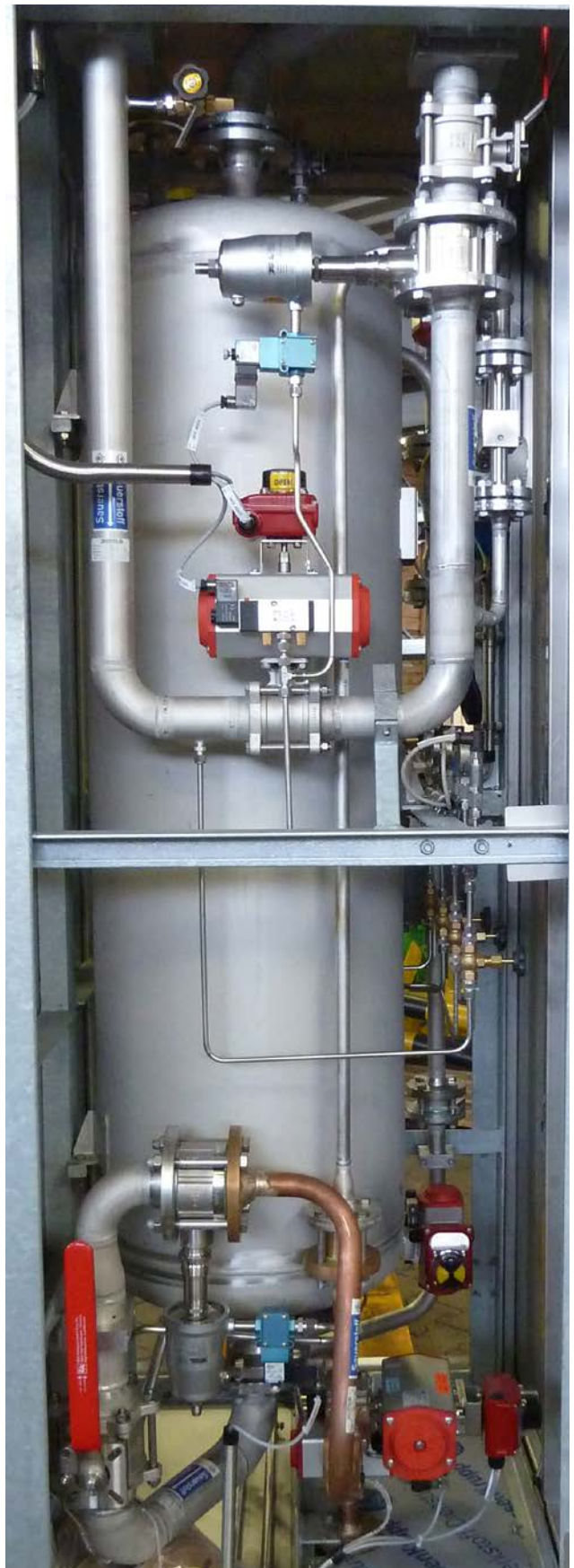
View inside an SIP box: Two type-8040 sliding gate valves were further developed over the years so that they are capable of releasing the necessary impulses with strong shock waves and have a minimum service life of one year, i.e. several million switching cycles.
